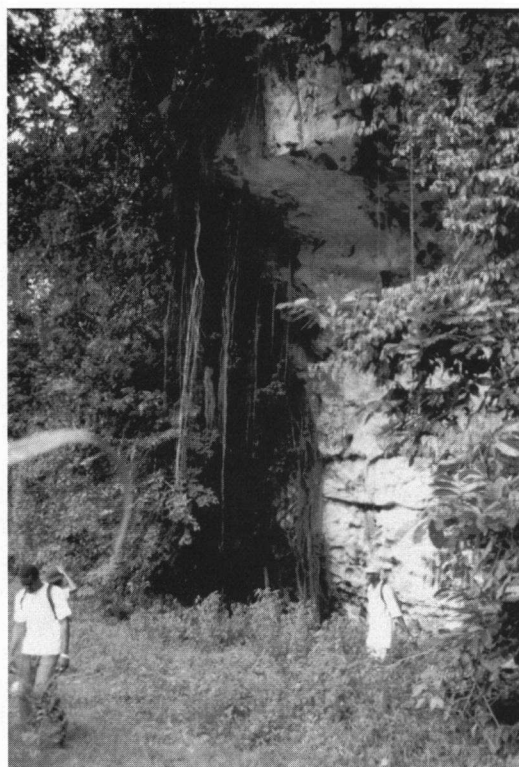
Figure 7. Tower in Troy Formation showing basal undermining, west of Lluidas Vale, parish of St Catherine.
